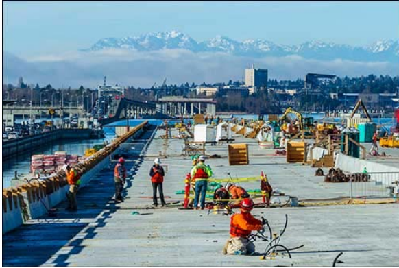
Construction of the new floating bridge, just north of the 1960s-era bridge, moves westward toward Seattle. (Jan. 2015; photo courtesy HDR)
